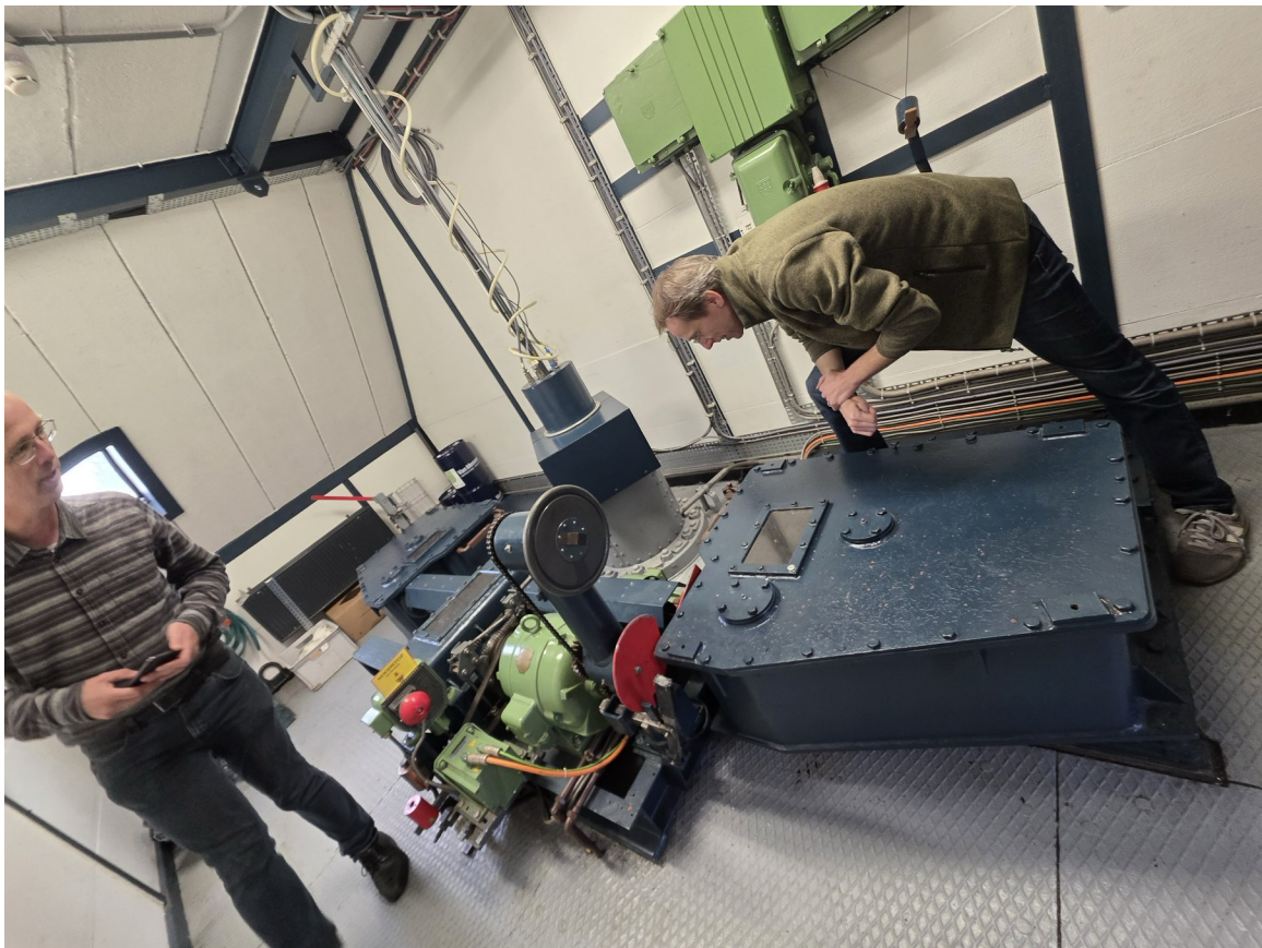
Fig. 3. Tammo Jan Dijkema (CAMRAS) and Thomas Telkamp (CAMRAS) inspect the main drive assembly after startup. The vertical shaft at top connects the rotating building to the stationary foundation; a monitoring system tracks cable wrap to prevent damage from over-rotation.
